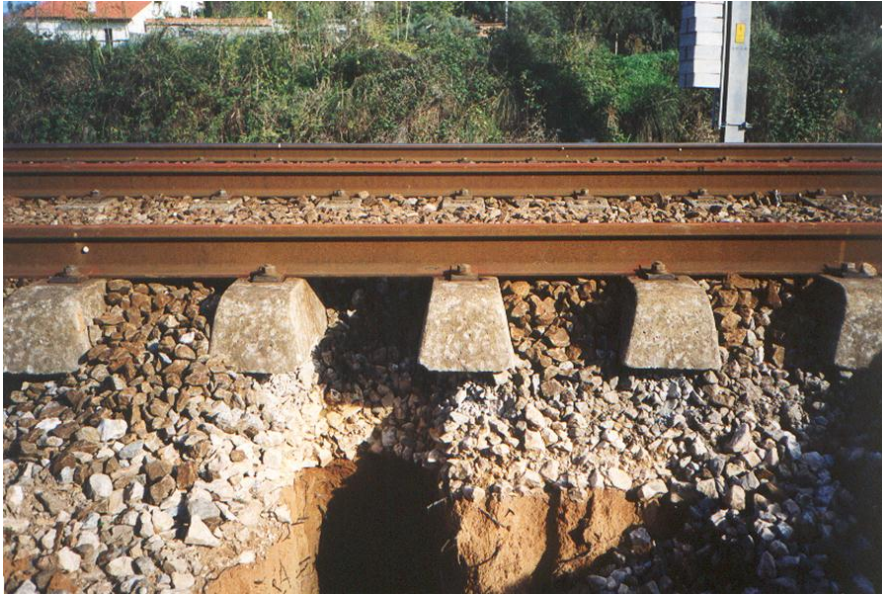
Figure 3.1- Example of degradation caused by fouling for a track formed by ballast and subsoil layers (Fortunato, 2005)
