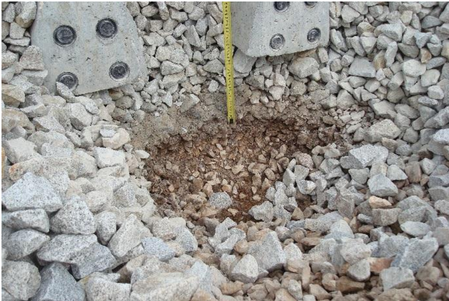
Figure 5.20 - Test pit with granite and limestone fouled ballast
