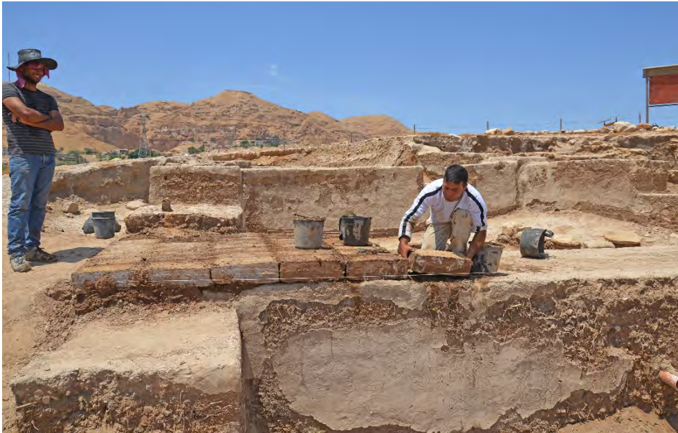
Fig. 21 - Training of a restorer laying bricks on the main wall of Palace G.
