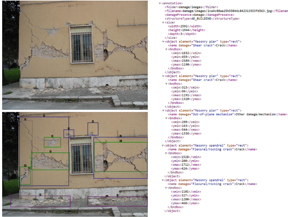
Figure 4.6. IDEA dataset: example of a typical building with instances of damage annotated using rectangular bounding boxes and polylines. On the right: content of the annotation file. On the left: original image (top) and annotated image (bottom). Image from [98]
