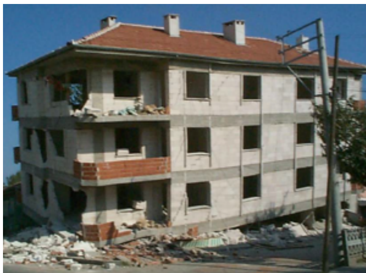
Figure 2.2. Damage level on building scale: (D4/D5) - Collapse or inclination more than 1%. Image from [5]
