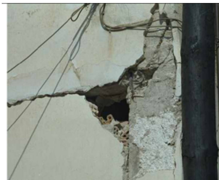
Figure 2.3. Damage level to single structural element (vertical structures): (D4) - Damage to the beam-column joint with concrete spalling and Crushing of the infill panel. Image from [5]
