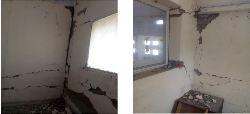
Figure 6. Cracks in column due to the presence of opening in infill (right) severe cracks in infill on the frame selected for analysis (left)
