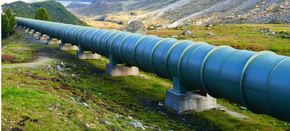
Fig 2: Water distribution network pipe
