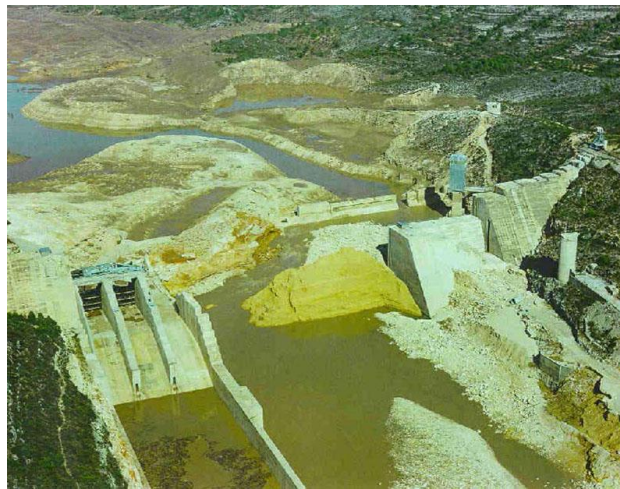
Figure 2.5 Original Tous Dam after overtopping failure (Photo source: Alcrudo, 2003).
