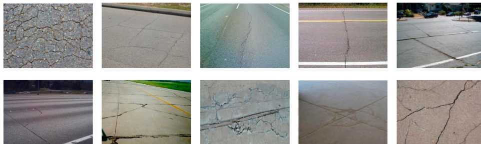
Figure 1. Some different crack types. In the top row (from the left to right: alligator cracking, block cracking, slippage cracking, longitudinal cracking, transverse cracking, and joint reflection cracking); on the bottom row (from the left to right: corner break, shattered slab/intersecting cracks, durability ("D") cracking, longitudinal, transverse, and diagonal cracking, and shrinkage cracks).
