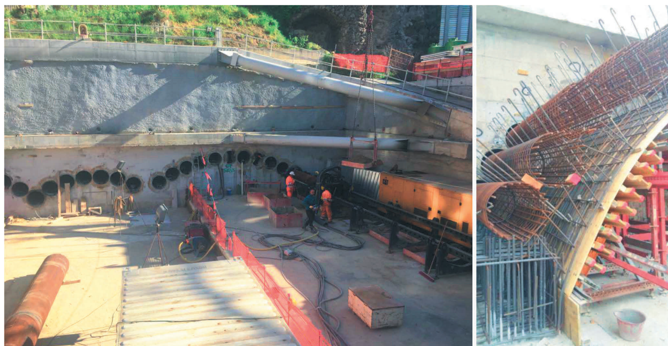
Figure 15. Steel pipes installed and steel bars in place for the connection with the entrance portal.
