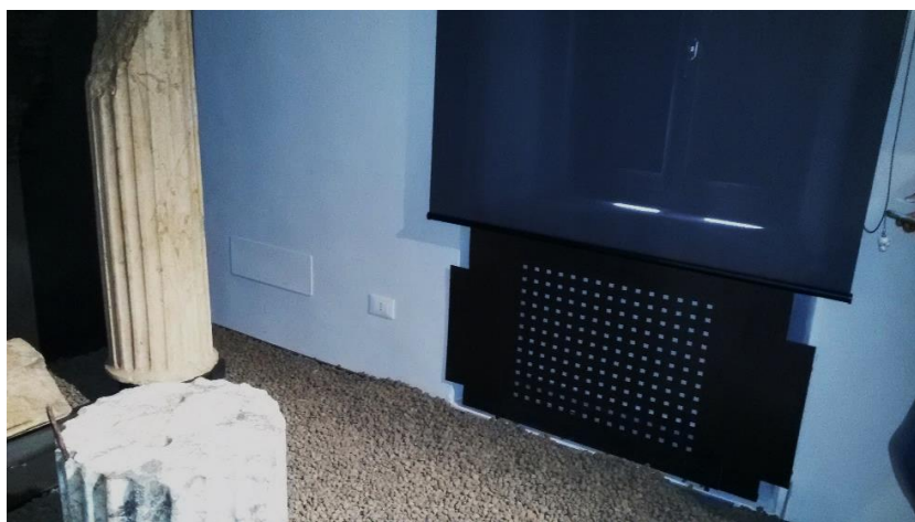
Figure 4 Black drilled-metallic panels cover fan coil installed under a window shaded by wooden shutters and a black roller blind.
