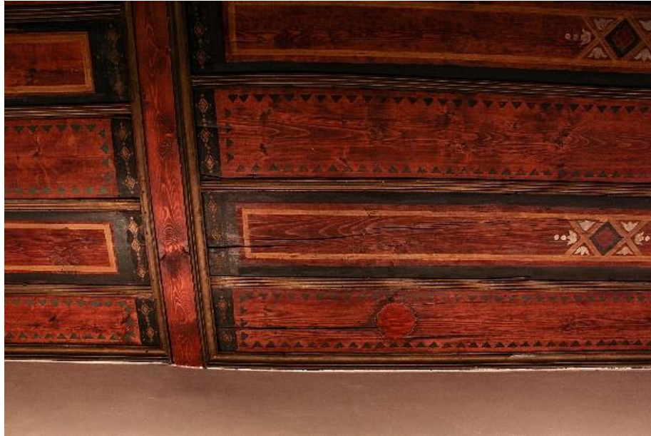
Figure 5 Details of the wooden ceilings decorated with oil paintings by Pietro Campeggi at the second floor. Cracks are visible along the tangential sections of wood.
