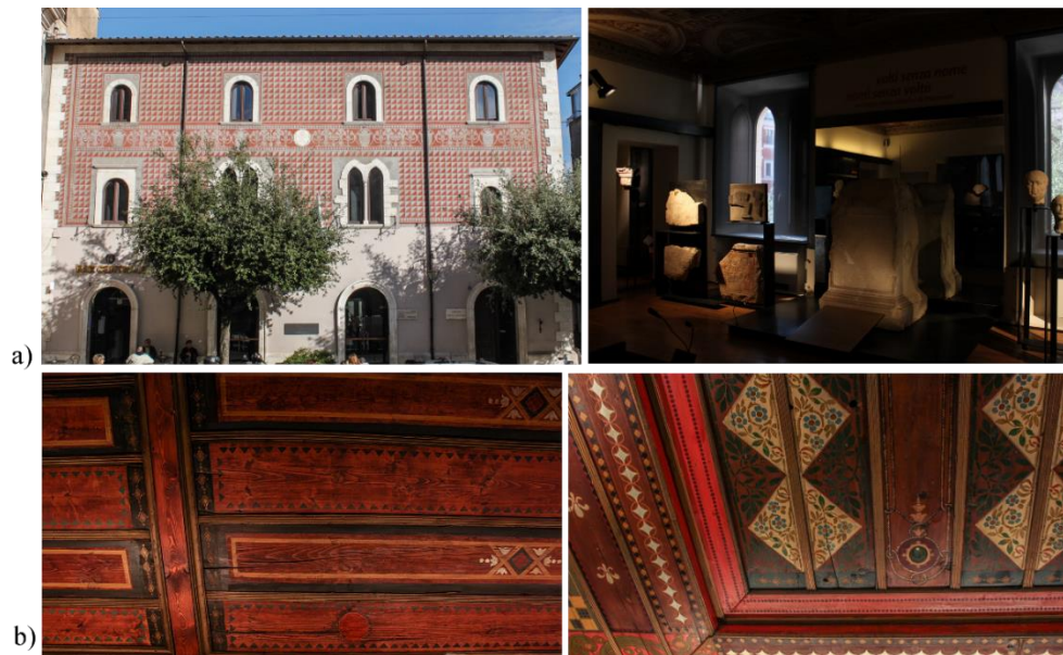
Figure 15 a) The “Museo Archeologico di Priverno”: outside (left panel) and inside (right panel). b) Details of the wooden ceilings decorated with oil paintings by Pietro Campeggi at the second floor. Cracks are visible along the tangential sections of wood.
