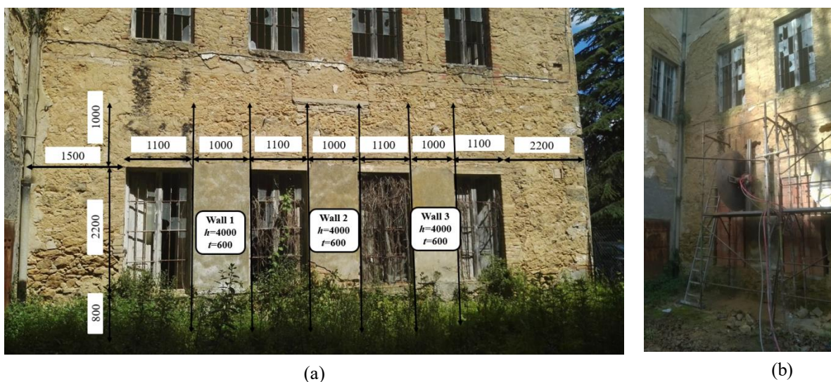
Figure 1 Tested rubble masonry walls: specimen identification and approximate measures in mm (a) and cutting process (b)
